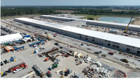
Google Data Center Campus, September 2024
